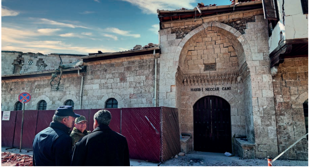
The historical Habib-i Neccar Mosque damaged by the earthquake
